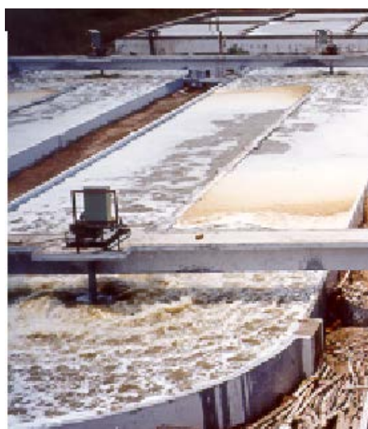
Fig.2: Oxidation ditches after the re-engineering
