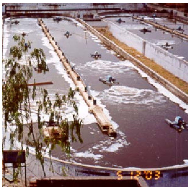
Fig.1: Oxidation ditches before the re-engineering
