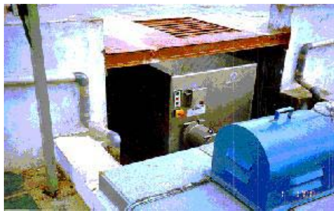
FRP coated platform from where fleshings is charged into the grinder
