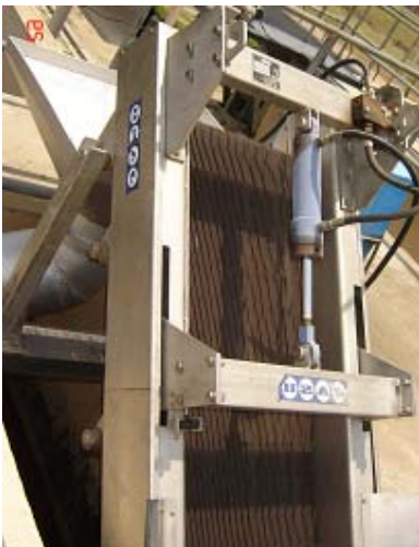
Picture 3 – New mechanical bar screen
