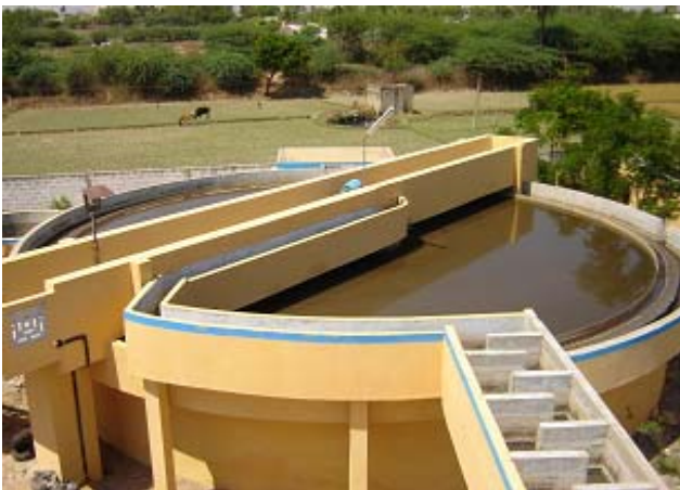
Picture 5 – Modified primary clarifier
