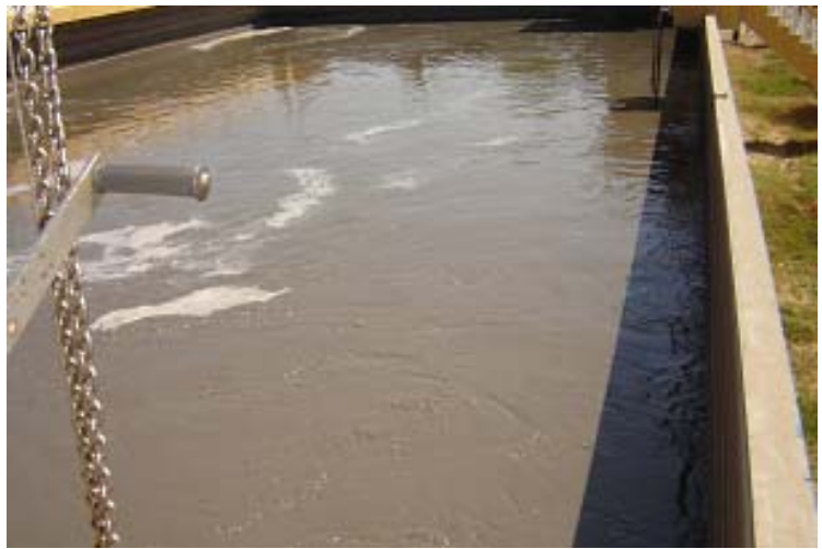
Picture 4 – Equalisation tank with new mixers
