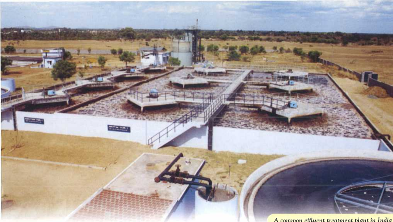
A common effluent treatment plant in India
